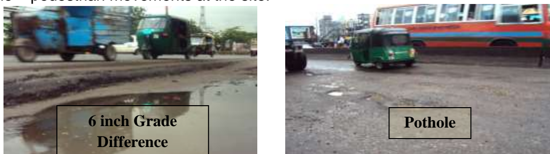
Figure-11: Road Surface Conditions (left- site-1 and right site-2)
